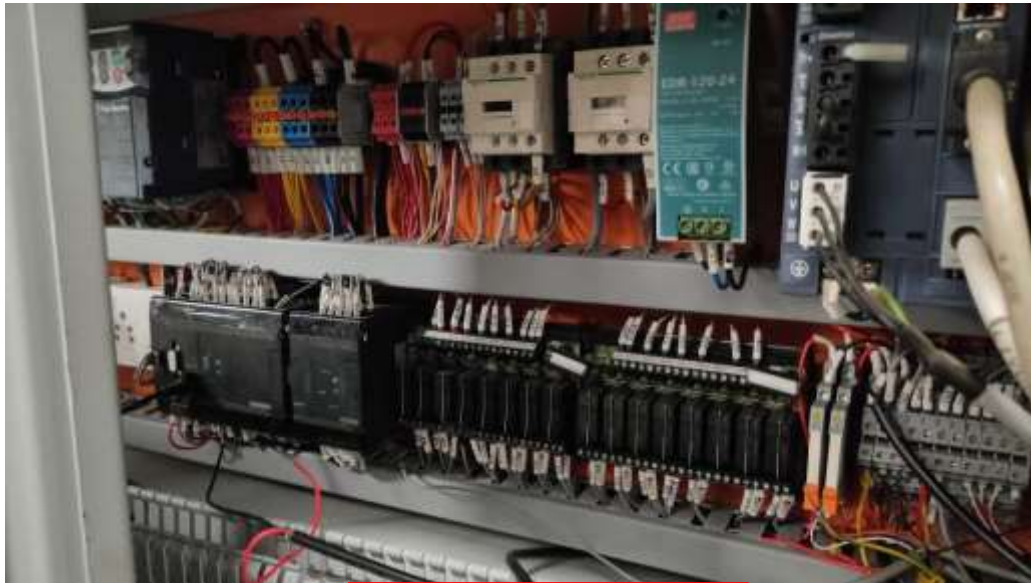
CONTROL PANEL IMAGE-1
