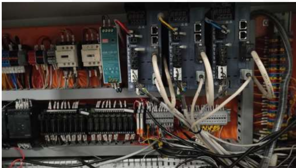
CONTROL PANEL IMAGE-2
