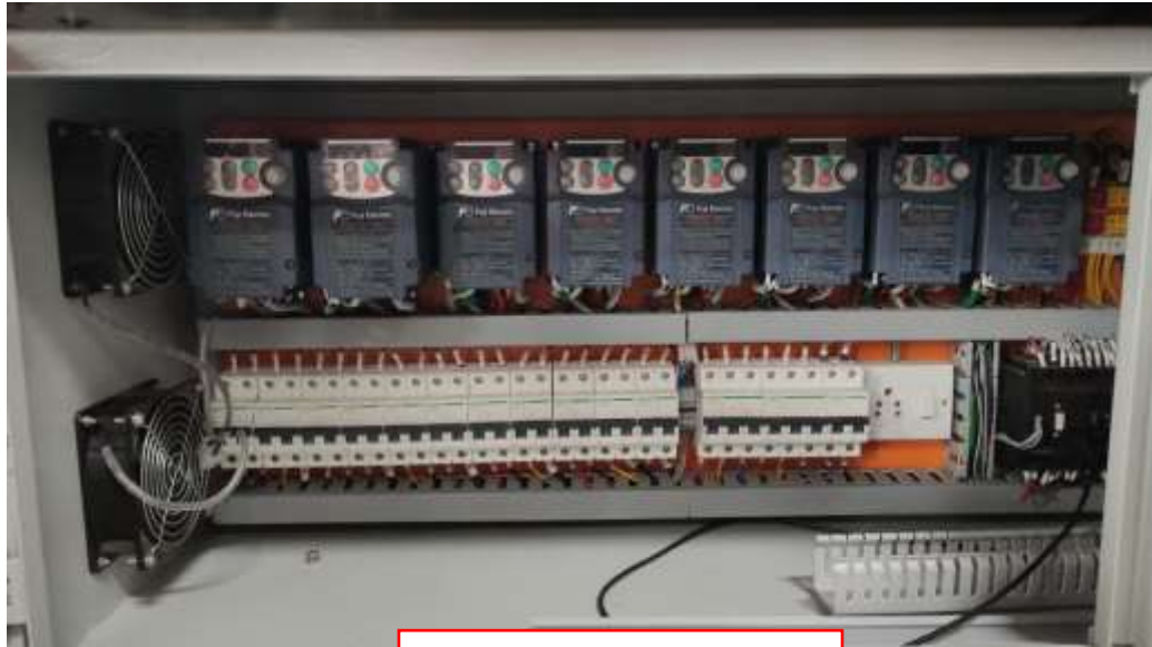
CONTROL PANEL IMAGE-3
