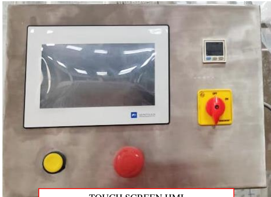
TOUCH SCREEN HMI FOR OPERATING & PROGRAMMING
